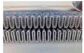
The Filter Media has absorbed water
